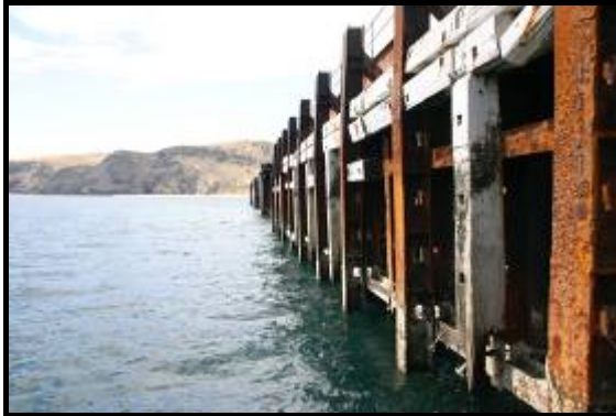
Decay of piles at seaward end of Jetty
